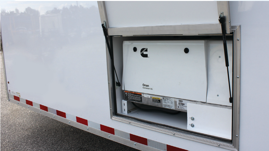
Commercial grade Cummins® ONAN generator
