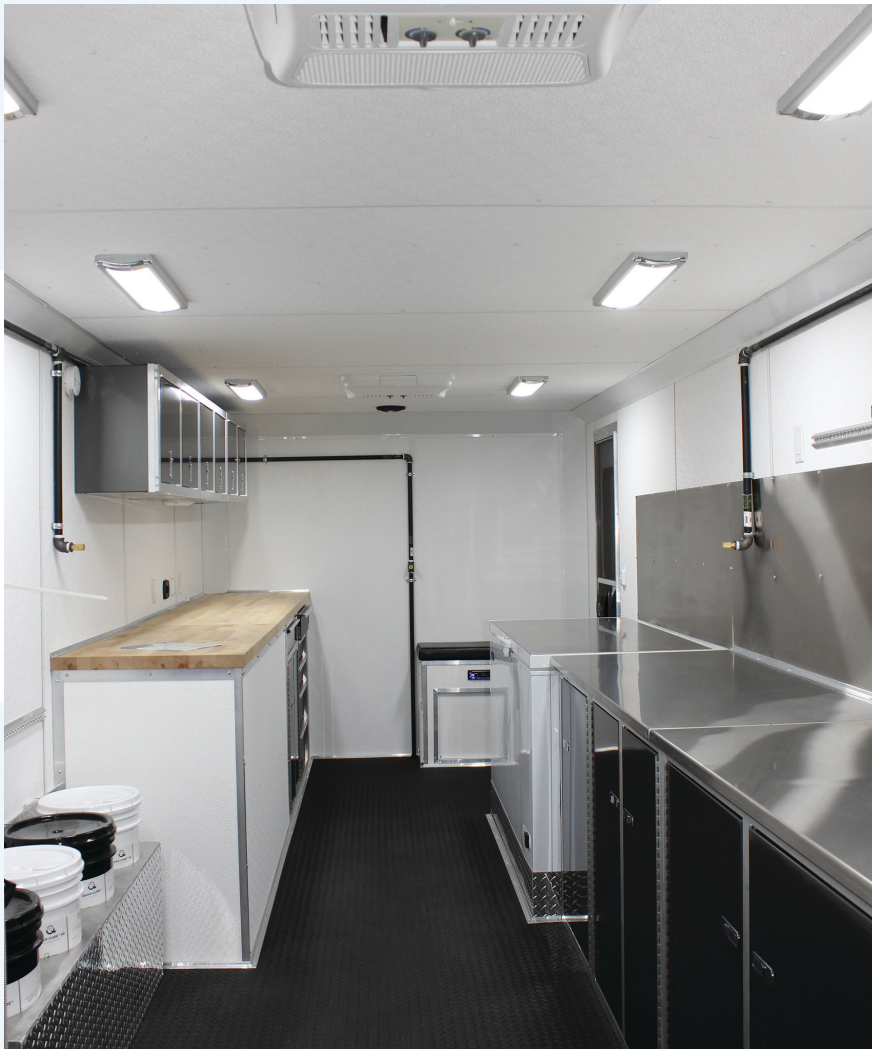
Dual ceiling mounted A/C system for comfortable working environment during summer season
